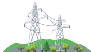
Transmission lines (110 - 800 kV)
